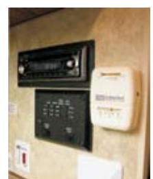
Control Center: • Monitor Panel (Holding Tanks & Batteries) • Generator Panel (optional - not pictured) • AM/FM CD/DVD (CD/DVD optional) • Solar Panel Monitor (optional - not pictured)
