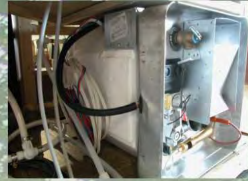
10 Gal. Water Heater
